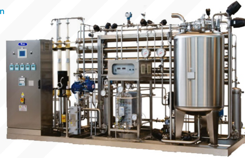
PURIFIED WATER GENERATION SYSTEM
